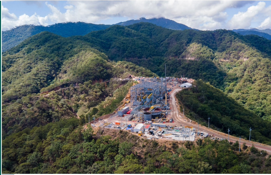
Erection of the assay lab and mill maintenance shop will commence in Q3.
