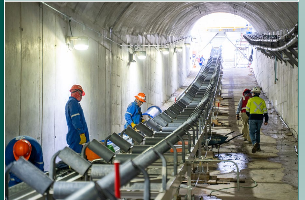
Inside view of the Coarse ore reclaim tunnel towards the grinding area
