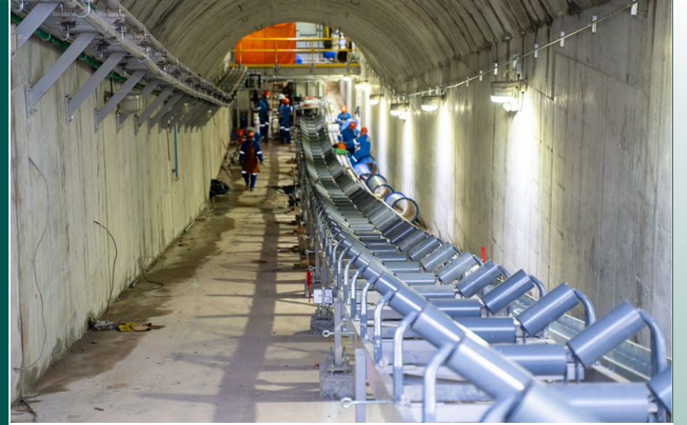
Inside view of the Coarse ore stockpile reclaim tunnel towards the feeder
