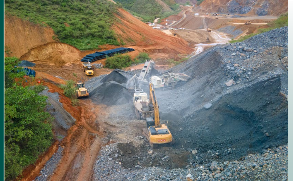
Drainage pipe ready for installation in July with crushed rock fill for tailing embankment
