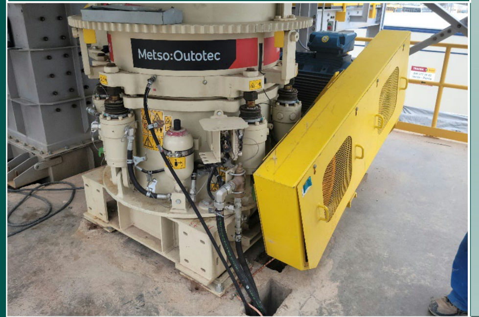
Grinding circuit pebble crusher
