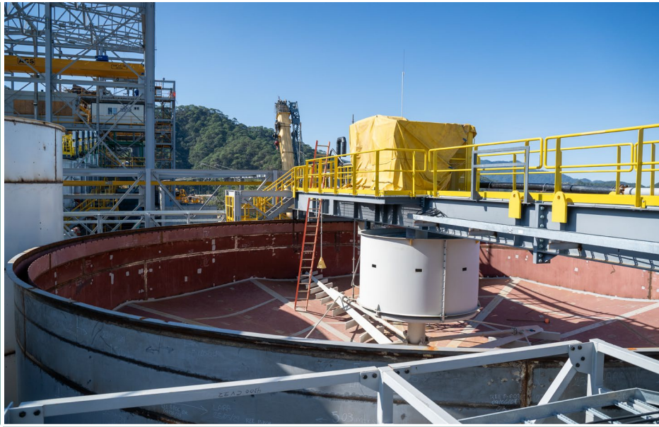
Tailing thickening tank
