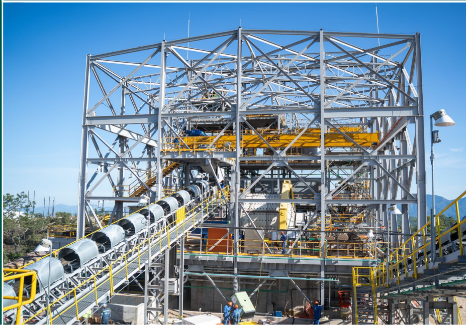
SAG mill feed conveyor from coarse ore reclaim tunnel
