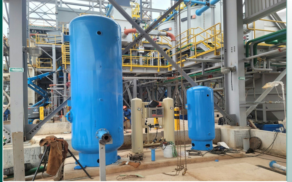
Compressed air receivers and air dryer system installed
